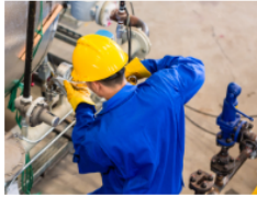
November 2020: Operations & Maintenance
